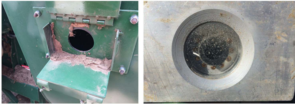
Figure 4 Mounting bracket used to mount the sensor on the air duct showing dust accumulation (left) and lens of the sensor located at that position showing abrasion and pitting from the pebbles and other foreign material.
